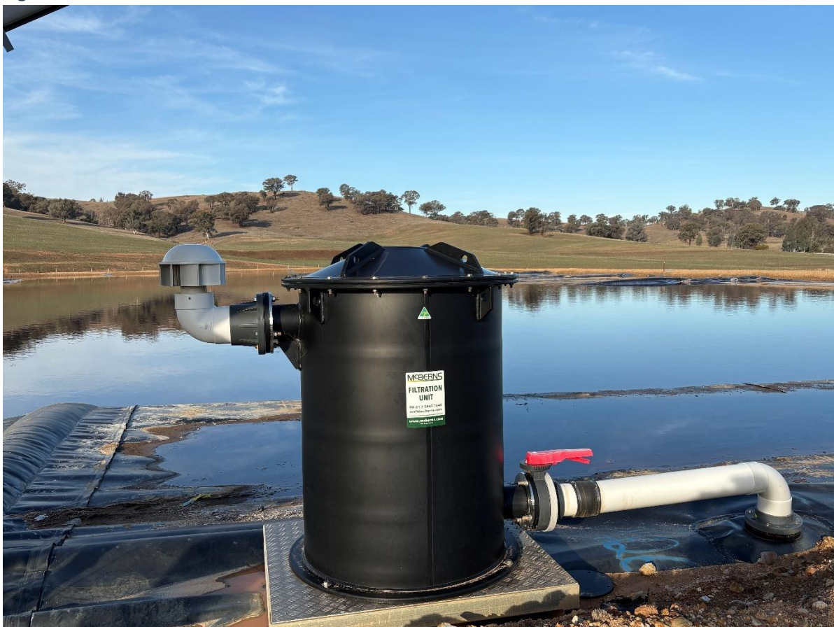
Figure 2 McBerns Odour Control Unit
